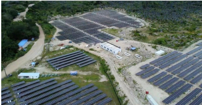
Solar farm site shared by the ADB and NZ government
